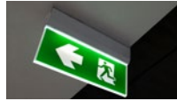
Exit signs and escape route lighting helps prevent panic and supports the safe, efficient evacuation of occupants by marking emergency exits, pathways, obstacles and changes of direction.
